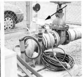
Deep well monitoring with Terminal box
