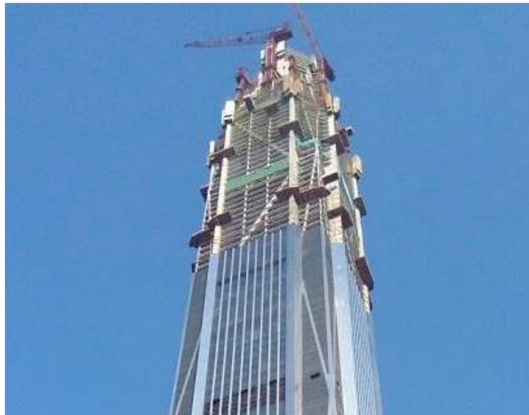
Figure 13. Ping An Finance Center during construction showing central core, two megacolumns on each side, perimeter diagonals, and belt trusses; outriggers are hidden inside (photograph in public domain).
