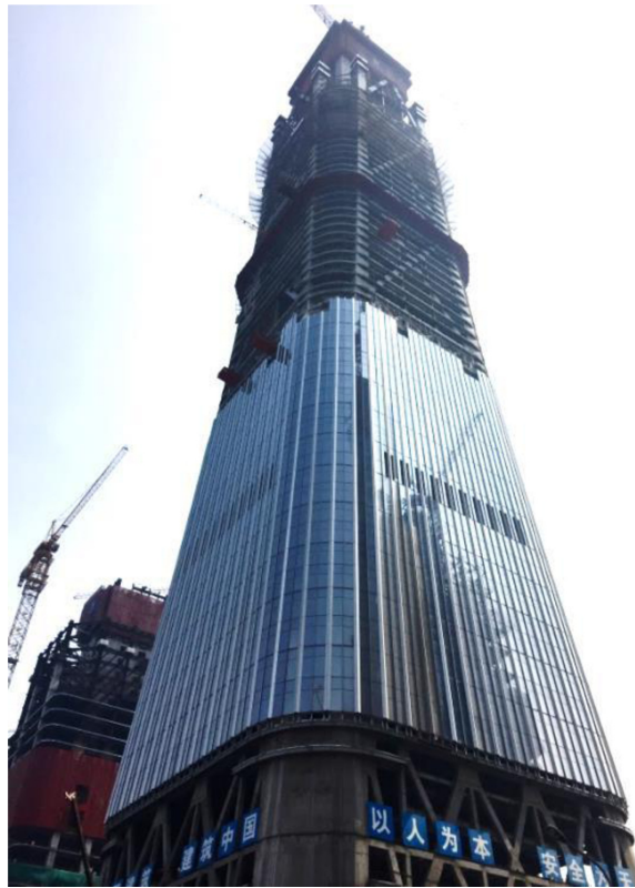
Figure 10. Citic Tower under construction showing single corner megacolumns on several lowest levels and split paired corner megacolumns on typical levels (photograph in public domain).
