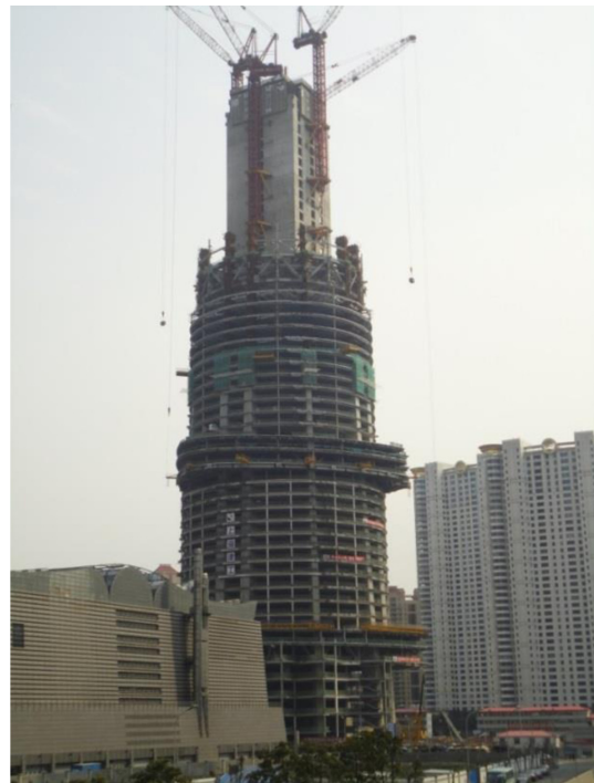
Figure 4. Shanghai Tower during construction showing central core, belt trusses and perimeter megacolumns (photograph by Kyoung Sun Moon).
