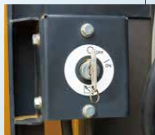
▲ Equipped with battery disconnect switch
