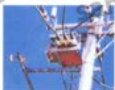
柱上真空開閉器 Pole-mounted vacuum switch
