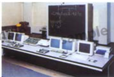
変電所総合運転システム Microprocessor based substation control system
