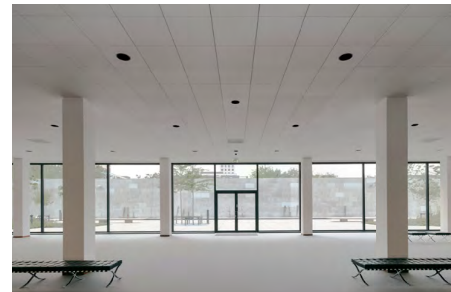
The need to comply with current fire safety regulations was the reason for improving and modifying the CEILING modules in the basement. A flexible ceiling system with metal cassettes now replaces the wooden substructure used during the original construction.
