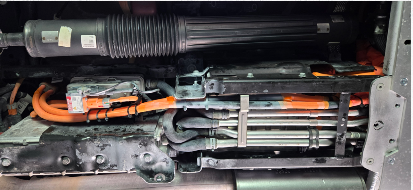
Image of the power pack skid-plate removed.
