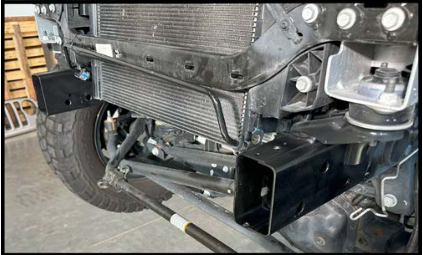
Step 15: Clean out the frame, deburr the holes and paint the frame in preparation for the final assembly.
