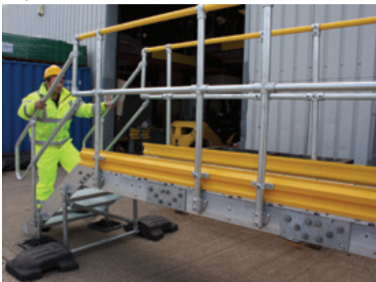
Handrail and toe-board to prevent falling of personnel and/or loose objects.
