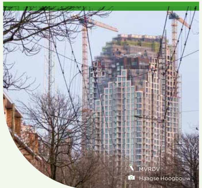
Grotius residential towers Closed cladding installed at the crown of the buildings - The Hague, the Netherlands
