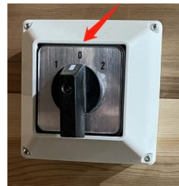
Power turned OFF
