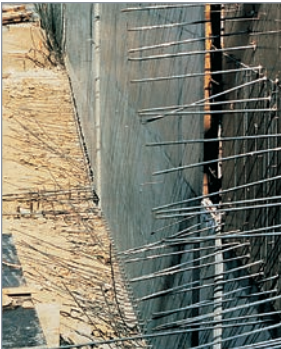
Exposed dowels on the job site are a hazard. In addition, they can be bent or damaged.
