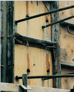
Drilling forms for dowels is expensive, and form removal is difficult and time consuming.
