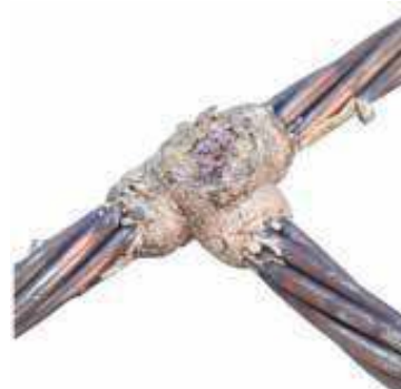
Reject. Excessive water in cable strands and/or mold.
