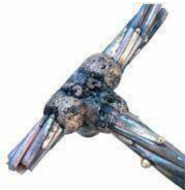
Reject. Heavy carbon coating on cable and connection is evidence of large amounts of oil or grease on cable. Cable must be cleaned with safety solvent.
