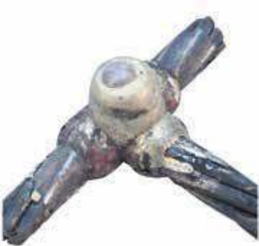
Reject. Light carbon traces on cable and connection are evidence of oil on cable strands. Oily cables must be cleaned with safety solvent.
