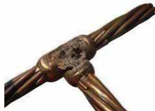
Reject. Fill too low. Weld cavity was not filled over cable strands. Absence of leakage indicates that welding material size was incorrect (too small) or thru conductor moved.
