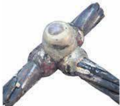
Reject. Light carbon traces on cable and connection are evidence of oil on cable strands. Oily cables must be cleaned with safety solvent.
