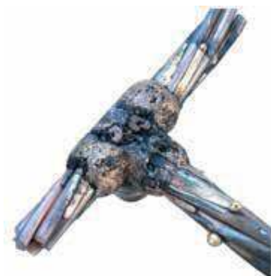
Reject. Heavy carbon coating on cable and connection is evidence of large amounts of oil or grease on cable. Cable must be cleaned with safety solvent.
