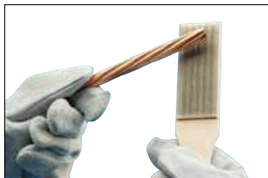
Fig. 12 Next, use a wire brush to further prepare the surface of the conductors (nVent ERICO T-313 or T-314 brush). Scrape the outer surface to remove dirt and oxidation. You will notice a slight color change.
