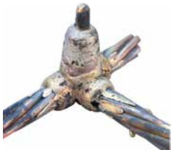
Good. A solid weld with only minor surface imperfections.
