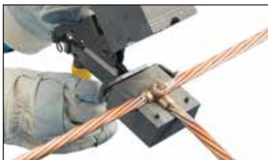
Fig. 22 Open the mold and remove the connection. Use care to prevent chipping the mold. Avoid contact with hot materials. See the “nVent ERICO Cadweld Quality Standards” section to see whether a quality connection has been made.
