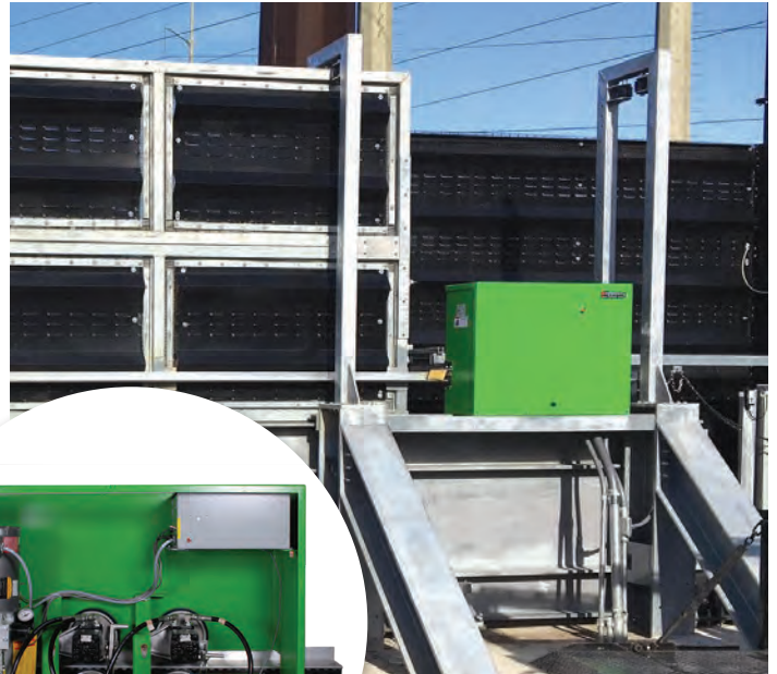
SlideDriver 200 operates crash gate at power substation
