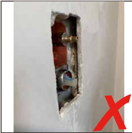
Valve installed too deep- incorrect installation
