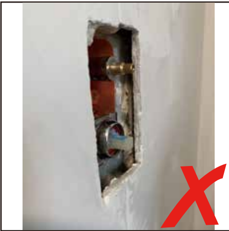
Valve installed too deep- incorrect installation
