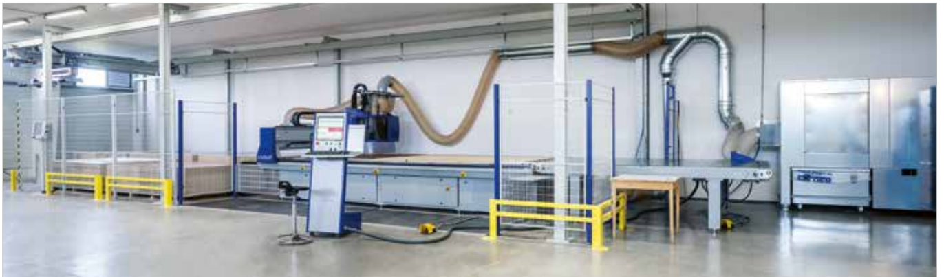
Automated milling center with feeder
