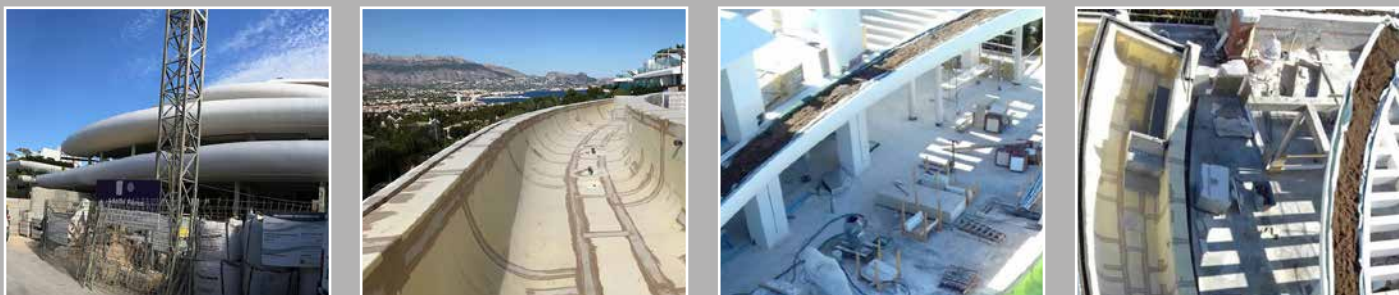
Waterproofing of outdoor swimming pools with DRY120 POOL . SHA WELLNESS luxury apartments. Albir (Alicante).
