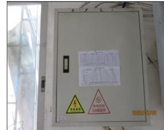
Photo of the inside of the main production hall electricity box.JPG
