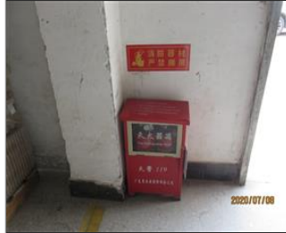
Photo of fire safety equipment fire extinguishers.JPG
