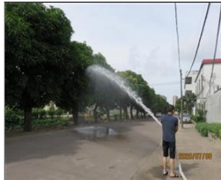
Photo of fire safety equipment fire hydrant testing.JPG
