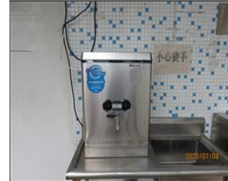
Photo of the sanitary facilities drinking water.JPG
