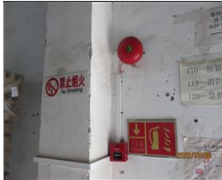
Photo of fire safety equipment fire alarm.JPG
