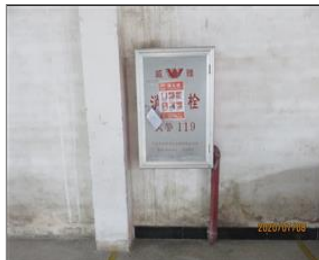
Photo of fire safety equipment fire hydrant.JPG
