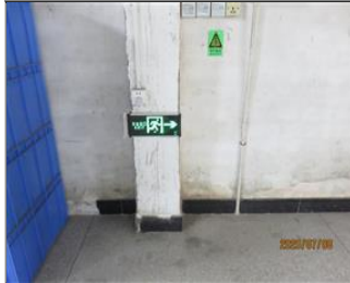
Photo of fire safety equipment evacuation sign.JPG
