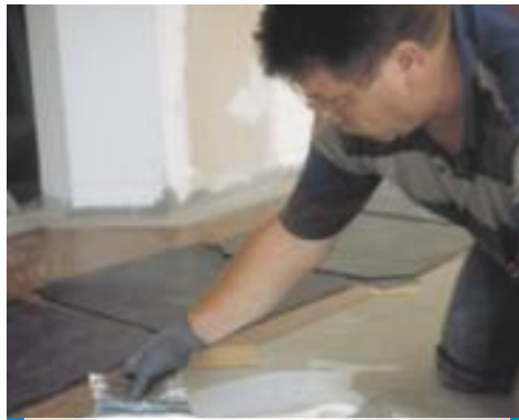
An example of an installation of inlaid PVC on a surface levelled with Ultraplan - CD2 - Milan - Italy
