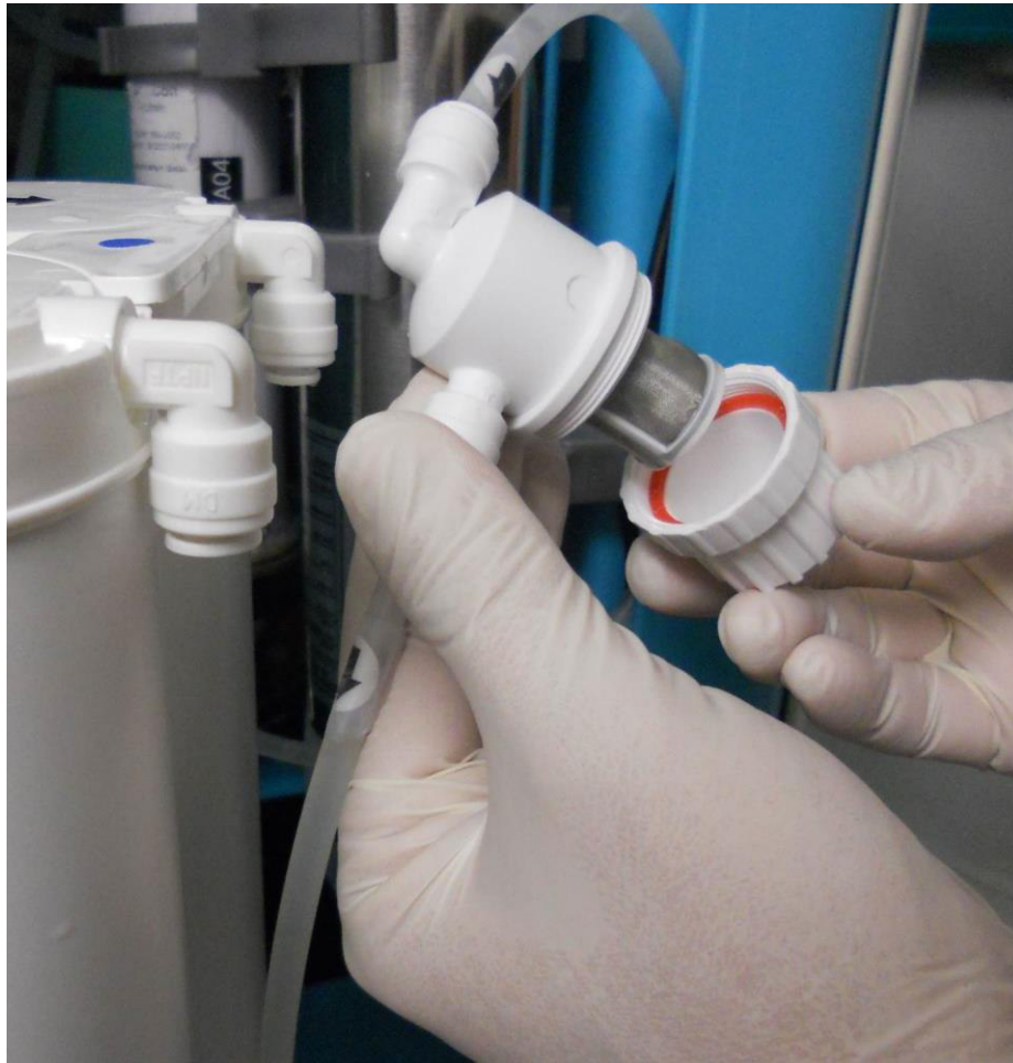
Figure 17: Disinfection cell with mounted strainer
