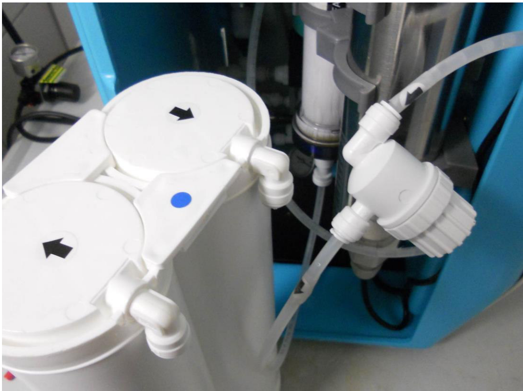
Figure 19: Mounted disinfection cell
