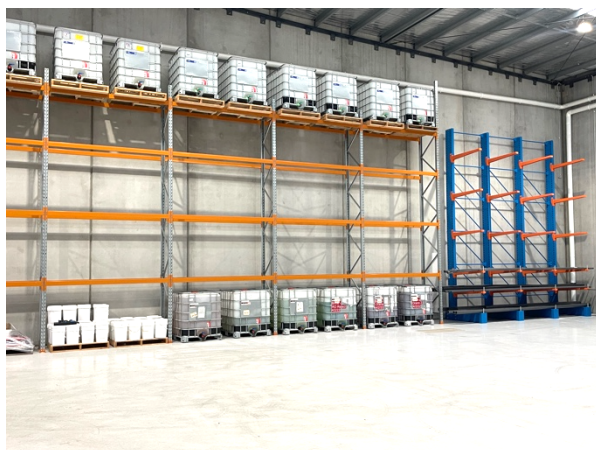
Figure 1c: Bulk salt and brine storage racking facilities.
