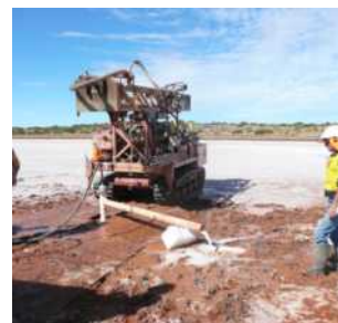
KLPP Brine Flow-Testing
