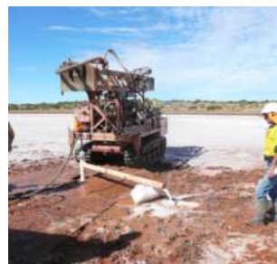
KLPP Brine Flow-Testing
