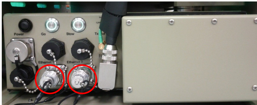
Figure 20: Tx and Rx Port on the Baseband
