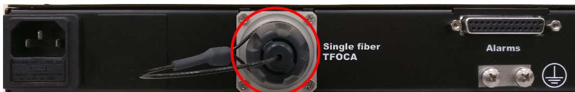
Figure 22: Fiber Optic Port on the Baseband
