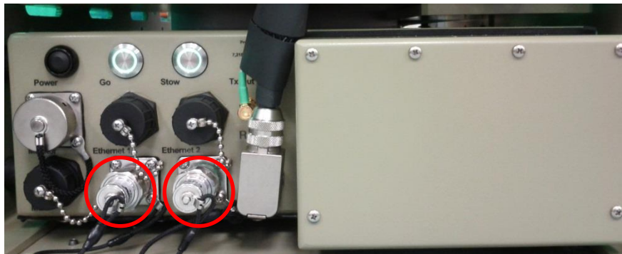
Figure 20: Tx and Rx Port on the Baseband
