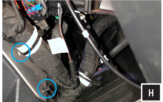
H. Remove the (2) push pins on the passenger side front of the center console.
