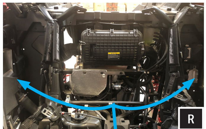
R. Route the B-H2195 Driver and passenger cables to their assigned speaker pods. Follow factory wiring harnesses when routing the cable and avoid sharp edges or rotating vehicle parts.
