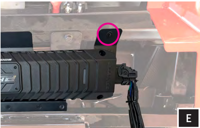
E. With the accurate location marked, uninstall the amp tray and use a 13/64" drill bit to drill your pilot hole. With your pilot hole drilled, reinstall the amp tray. Use the self-tapping screw in the drilled hole location.
