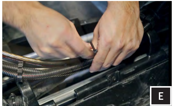
E. Zip tie all of the electrical cabling (factory and audio) along the center column away from the drive shaft.
