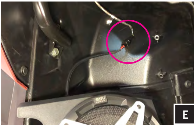
E. Connect the B-H1909 cable to both passenger and driver side speaker pods and zip tie all cables to the frame.
