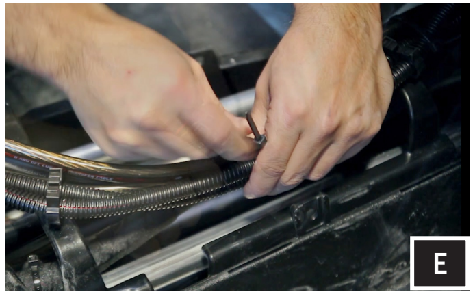
E. Zip tie all of the electrical cabling (factory and audio) along the center column away from the drive shaft.
