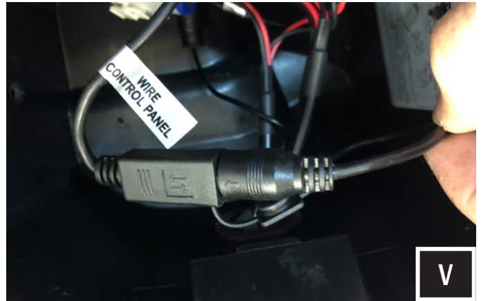
V. Align the arrows on the wire control panel with the arrow on the MRB3 controller connector and connect.
