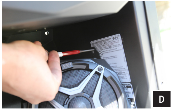
D. While holding the pod in place, use a scribe to mark a drill point for the pilot hole.
