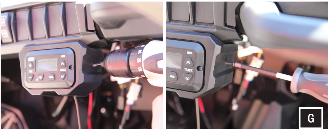
G. Drill a pilot hole on either side of the DM3 with a 3/32" drill bit. By hand fasten down using the (2) #6x.5" screws.
