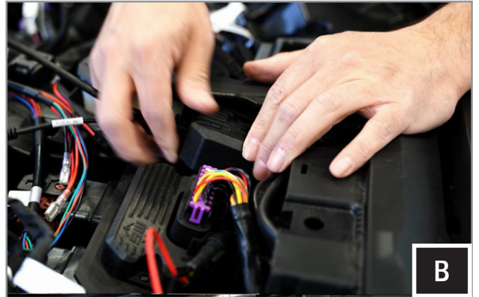
B. Mount the LIT-CC RGB LED Controller Command Center in the dash away from moving parts and secure with zip ties. Cut excess zip ties for a clean install.
