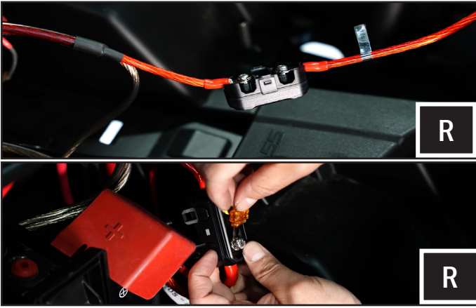
R. Install the fuse holder on the power wire no more than 18" away from the battery and install the fuse.
