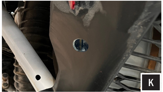
K. Drill a 3/4" hole in the rear of the vehicle for the turn signal LED lamps. Refer to the viewing angle diagram on page 7 for proper turn signal LED lamp placement.
