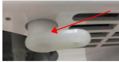
Cold Steam Drainage
