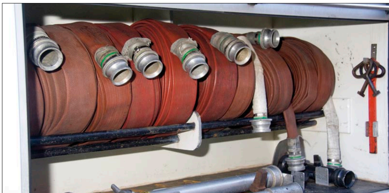
Figure 39 Firefighting hoses conspicuous locations along the escape routes, such that nobody in the storage area needs to travel more than 30 metres to reach one. Unless the location of an extinguisher is self-evident, its position needs to be identified by appropriate safety signs. Such signs should comply with the Health and Safety (Safety Signs and Signals) Regulations 1996 or BS 5499-1. 53
