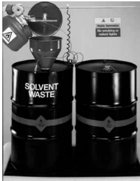
Figure 2 Example of system for waste solvent collection
