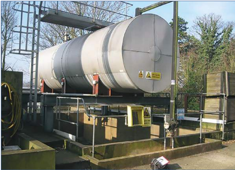
Figure 6.4 Example of installation vulnerable to jetting of fuels over the bund wall (courtesy CH2M Hill, with permission from the Environment Agency)
