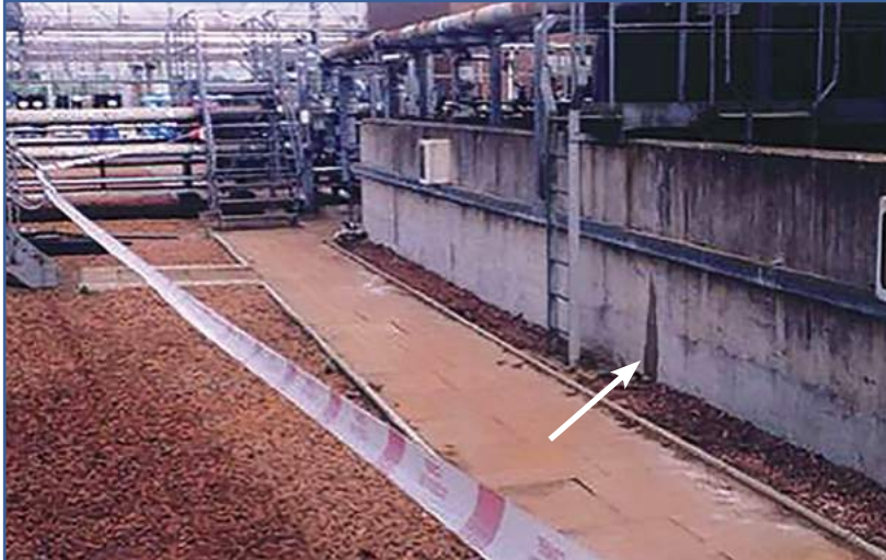
Figure 5.2 Arrow shows leaking crack in a bund wall (courtesy CH2M Hill, with permission from the Environment Agency)
