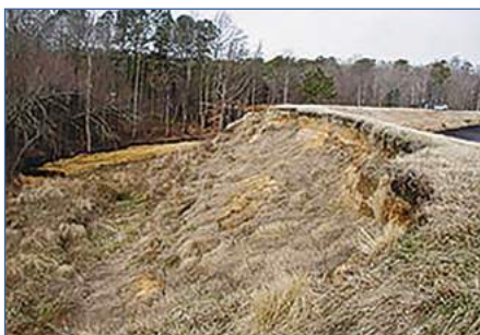
Figure 5.5 Slumping of earth embankment
