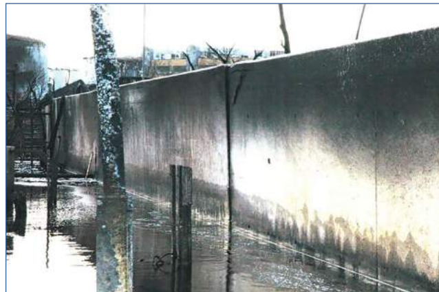
Figure 5.12 A joint that has failed due to thermal expansion because of inadequate dowel provision across the joint. Note also that the tie bolt holes at the foot of the wall also leaked during the incident (courtesy CH2M Hill, with permission from the Environment Agency)
