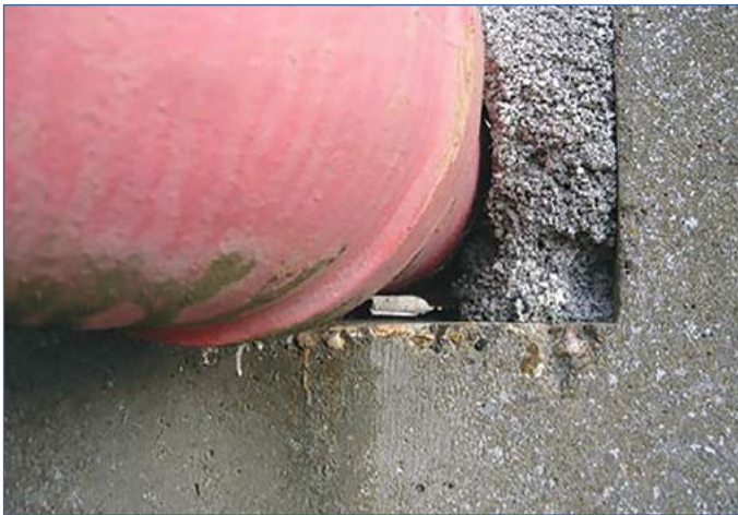
Note the pipe is bearing on the formed hole such that the infill concrete or mortar beneath will not form an adequate seal. In addition there is no puddle flange on the pipe.
