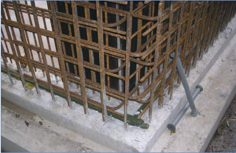
Figure 5.13 A kicker joint (note the use of hydrophilic sealants is not recommend)
