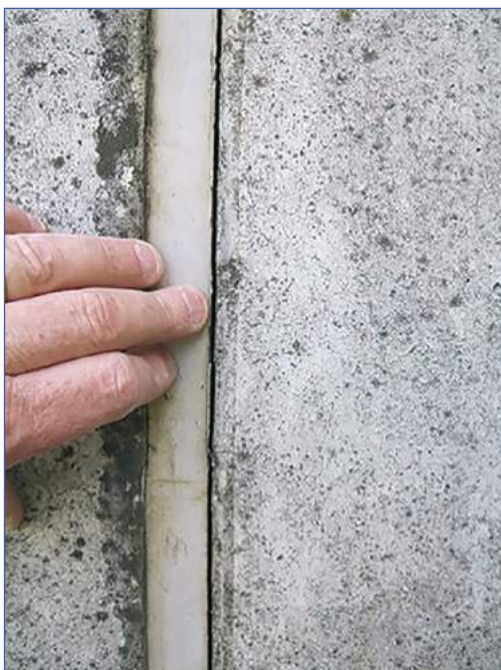
Figure 5.15 Over time, sealants will detach from the sides of joints and must be regularly inspected and replaced (courtesy CH2M Hill, with permission from the Environment Agency)
