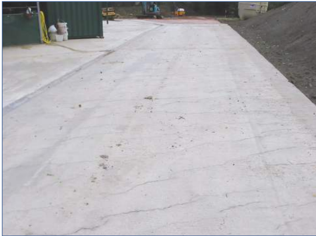
Figure 7.6 Plastic shrinkage cracks (courtesy Concrete Society)
