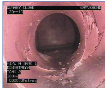
Figure 5.7 CCTV survey equipment and of a defect in a pipe (courtesy InSewer Surveys)
