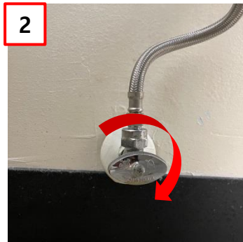
② Close the water valve clockwise
