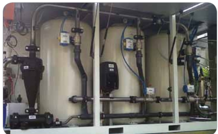
• EURO MEC water treatment plants "Progetto H2Ohhh!" Pomabamba, Peru. Chemline Hydro Cyclone shown on the left. Photo courtesy of Euro Mec.
