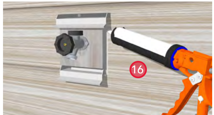
16. Apply sealant around the perimeter of the face plate and sill flashing (bottom and sides).
