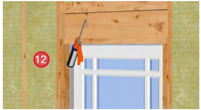
12. Install backer rod and sealant around the interior perimeter of the door frame to maintain air barrier continuity.
