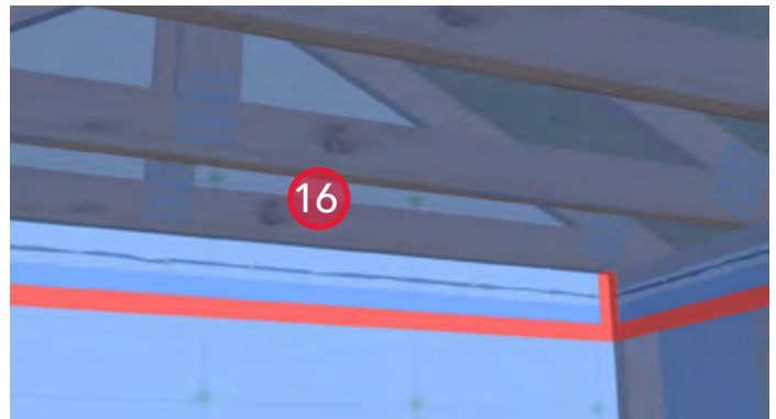
16. Install poly to the underside of the roof framing and fasten with staples at the sealant bead to complete the air seal. Seal the leading edge with sheathing tape.
