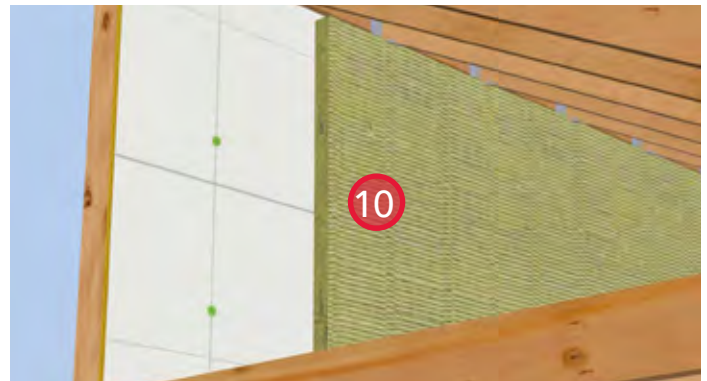
10. Install ROCKWOOL COMFORTBOARD™ 80 on the exterior of the wall between canopy ledger boards with recommended fasteners.
