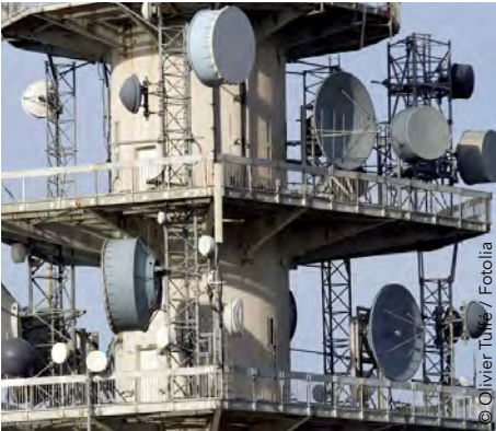
Telecom - Data infrastructure
