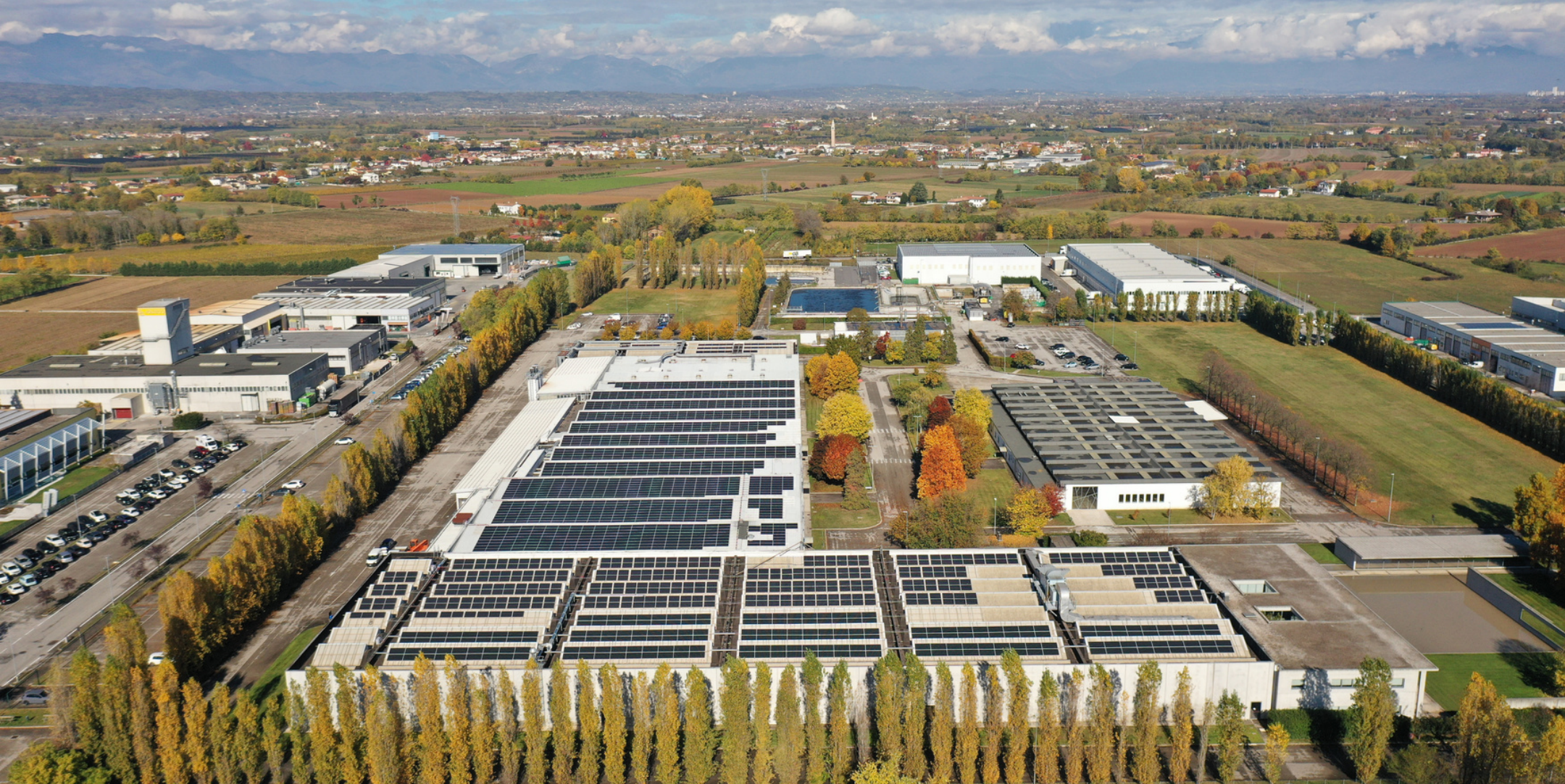
Photovoltaic system on Ponzano Veneto (TV) plant
