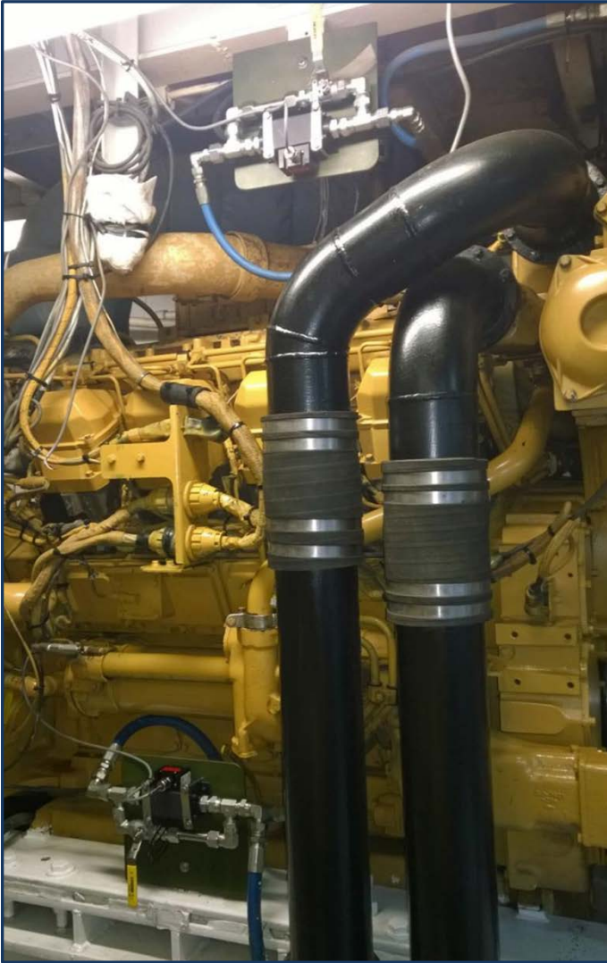
Port Main Engine Caterpillar 3508B Rated at 1100hp
