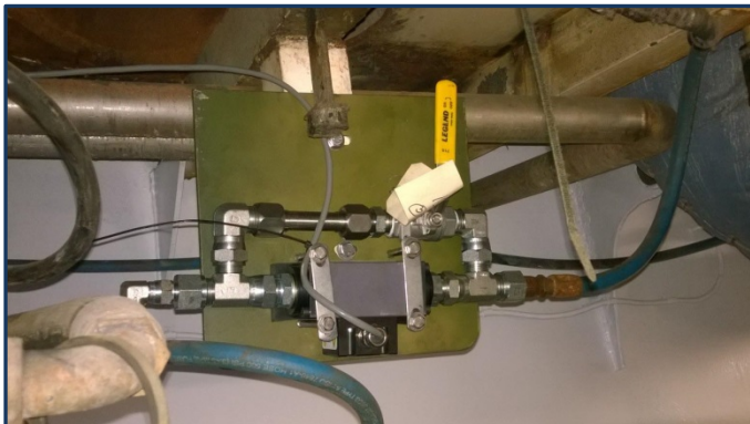
Port Main Engine with Kral OME20 Return Fuel Flowmeter
