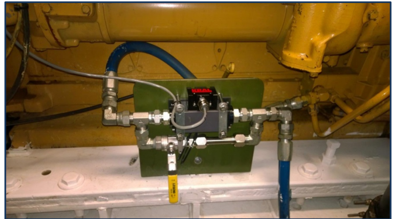
Port Main Engine with Kral OME20 Supply Fuel Flowmeter
