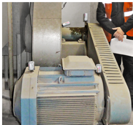
A combustion fan lubricated with two 60 ml and two 125 ml simalube lubricators.
