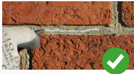
Fig 3. Mortar with scratch mark
