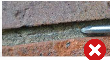
Fig 4. Mortar without scratch mark
