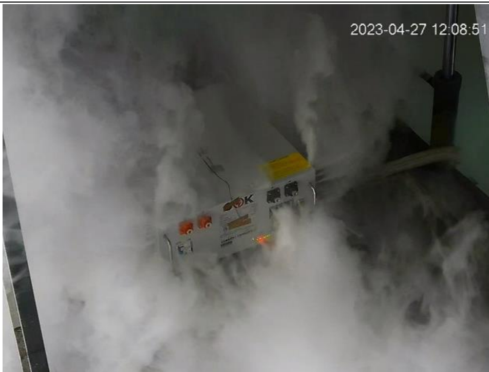
Thermal runaway observed
